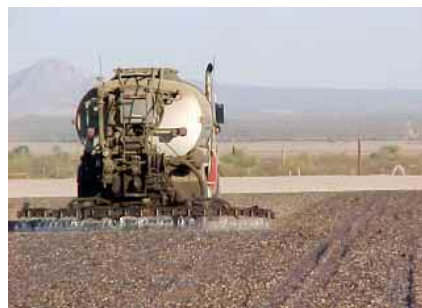
EnviroKleen® is sprayed on the native soil with trucks designed for this task.
